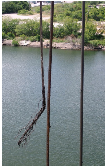
Parted wire rope on the crane side
