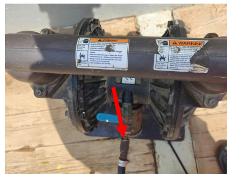
Disconnected hose end connection
